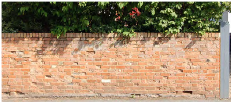
Picture 1.20 Spalled brickwork on the wall between Chestnut House and No.2 The Cottages detracts from the overall quality of the streetscene. Remedial action would be desirable
